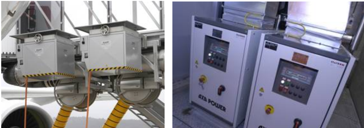
Figure 3 Cable and hose coils (left) and 400Hz transformers (right)
