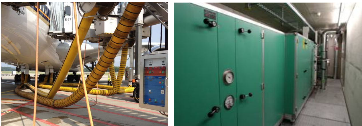
Figure 5 Hose for pre-conditioned air (left) and central PCA plant (right)
